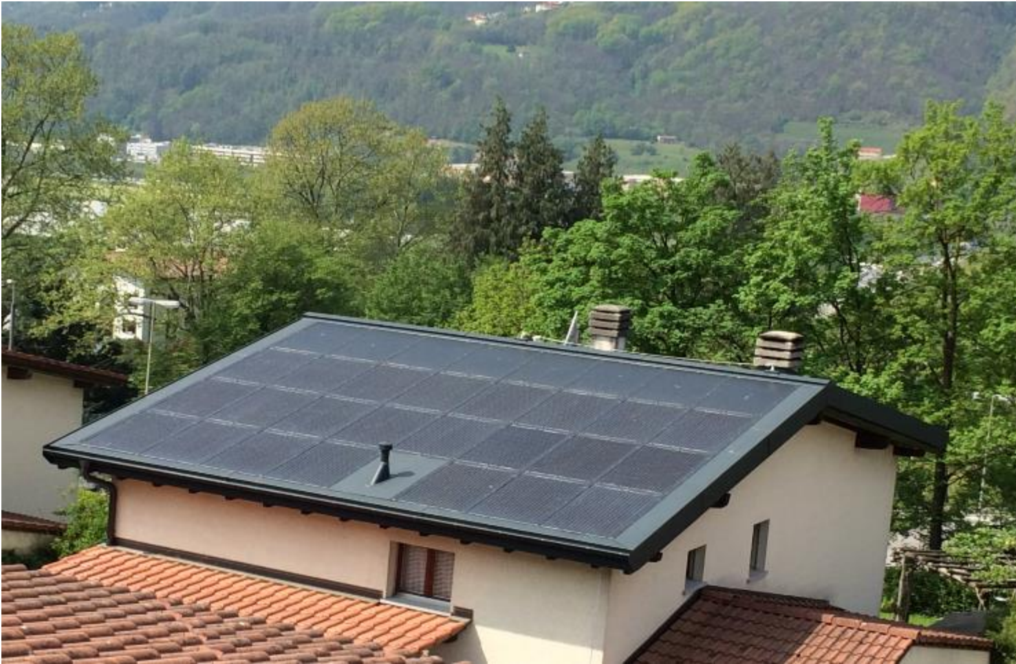
100 sqm, 7 kWp, Switzerland - Residential
